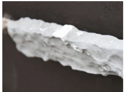
Anode Needing Replacement
